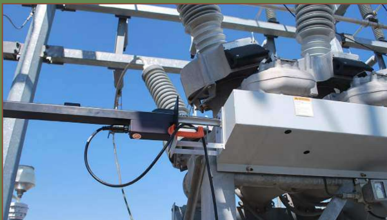
25" transducer on Siemens SPS2 Breaker
